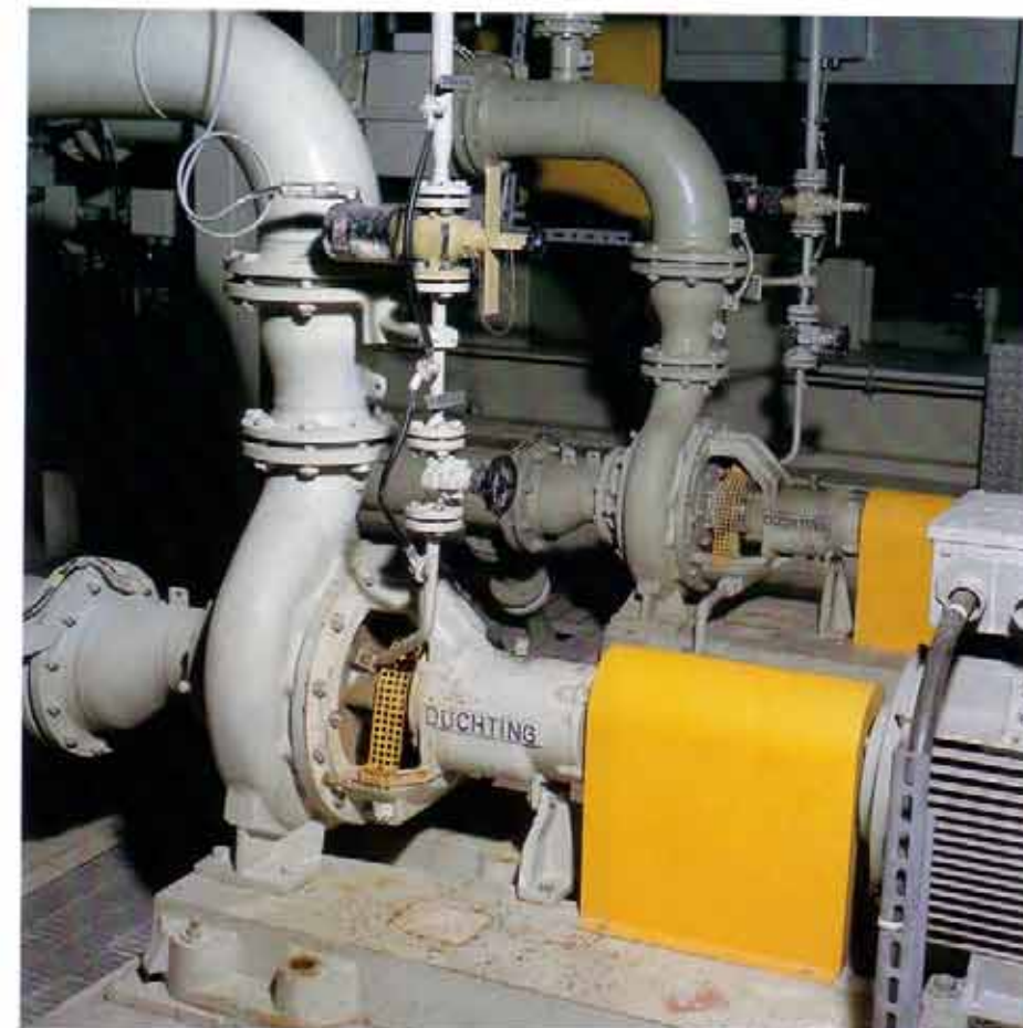
ROWA-E 80.40 Handling gypsum-slurry in a flue gas desulfurization plant
